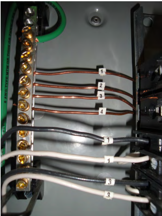
Ground Wire Bus on the Left
