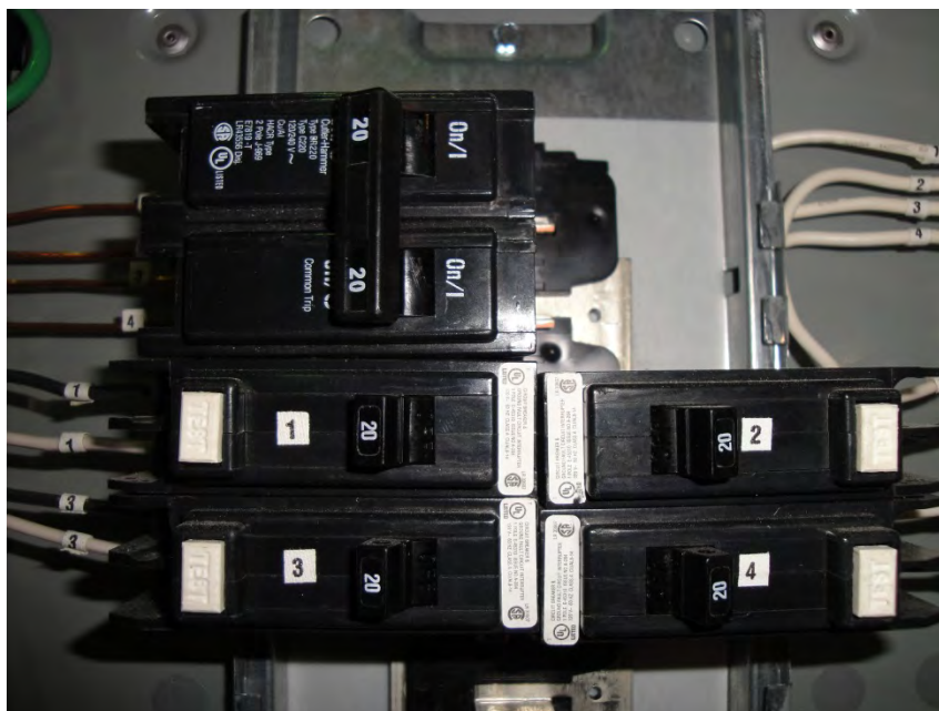
MAIN and #1, #2, #3 and #4 GFCB Circuit Breakers
